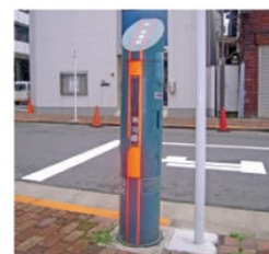
Green: Fire extinguisher managed by Taito City
